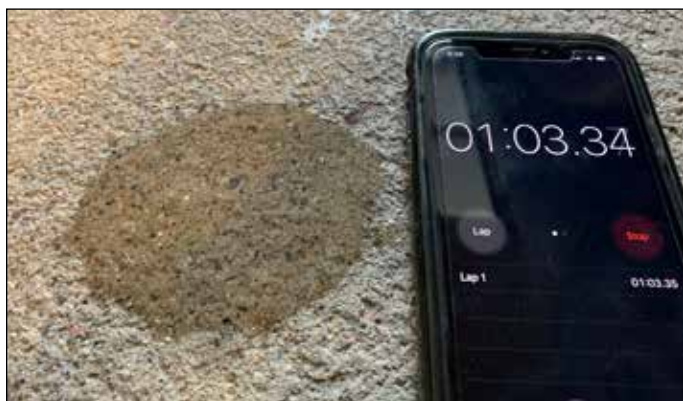
Figure 1. Water droplet partially absorbed after 1 minute indicating concrete is porous
