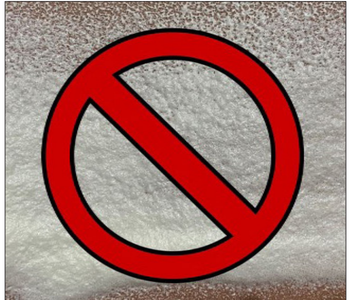
Image 2: Improper adhesive application
