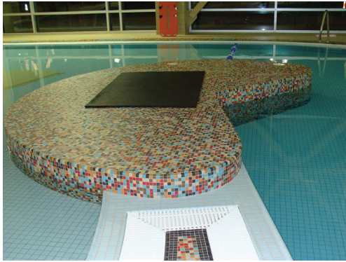
100% silicone caulk and a high-performance grout and mortar were used on this demanding installation.
